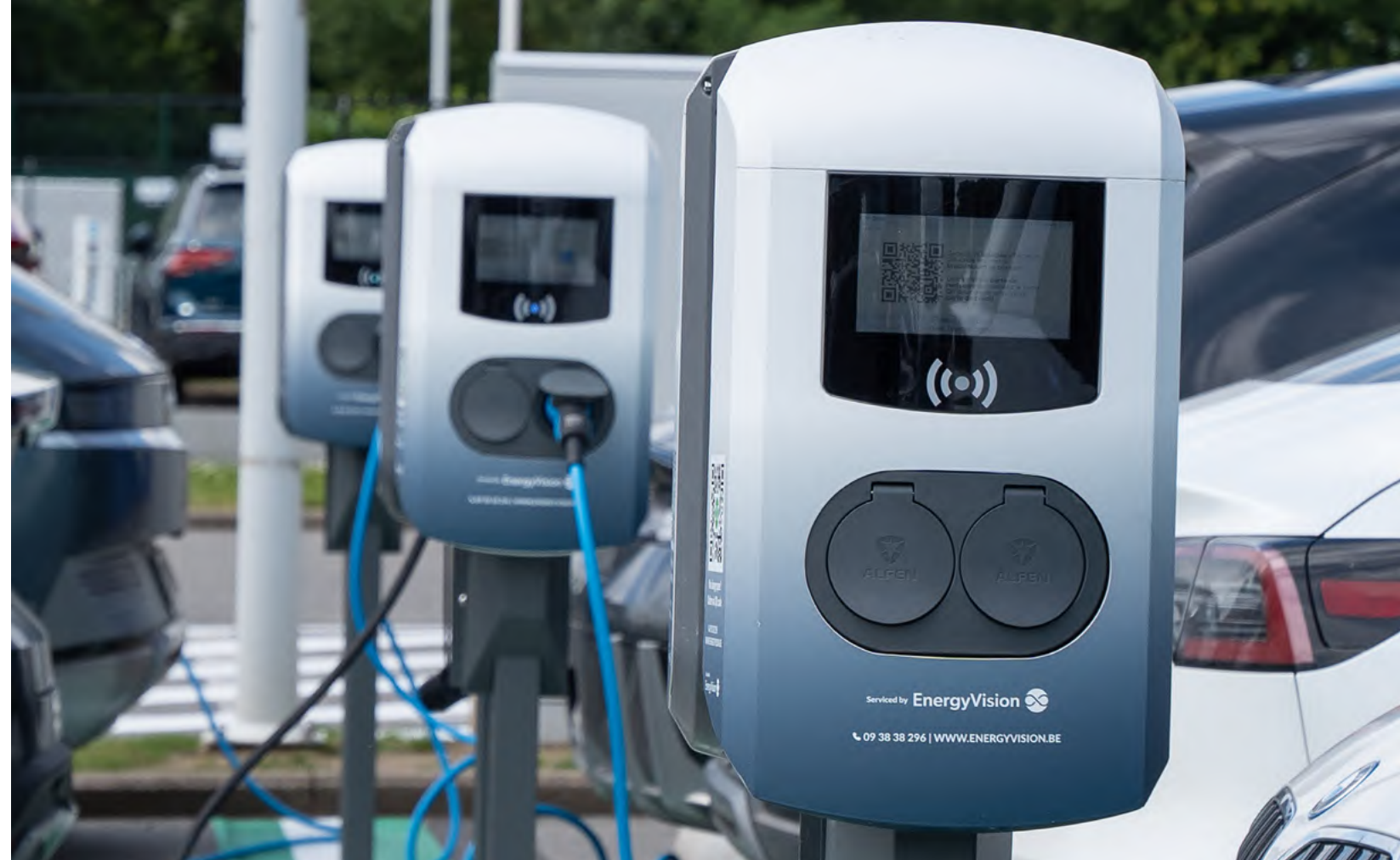
AC-laadpalen op de parking van Planet Group Arena in Gent, serviced by EnergyVision.
