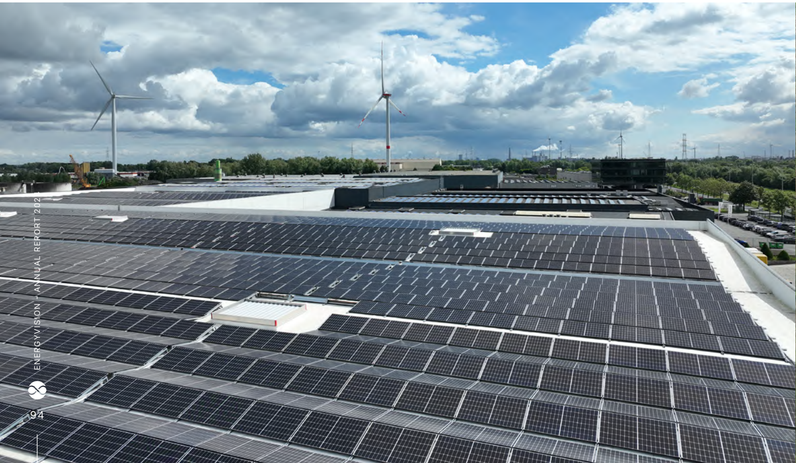
✓ Solar installation with 3,790 solar panels on the roof of Laroy Group in Wondelgem.
