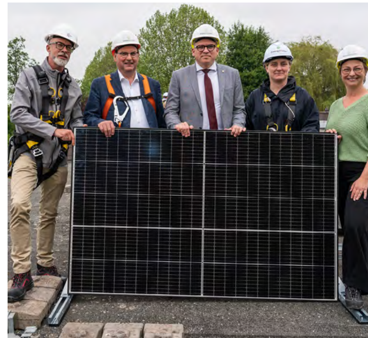
Flemish Minister for Housing Matthias Diependaele (middle) installs the 30,000th ASTER solar panel on one of the roofs of a social housing neighbourhood in Oudenaarde.
